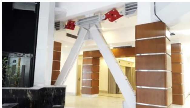
Figure 4. View of Rotational Friction Dampers in Chevron Bracing
