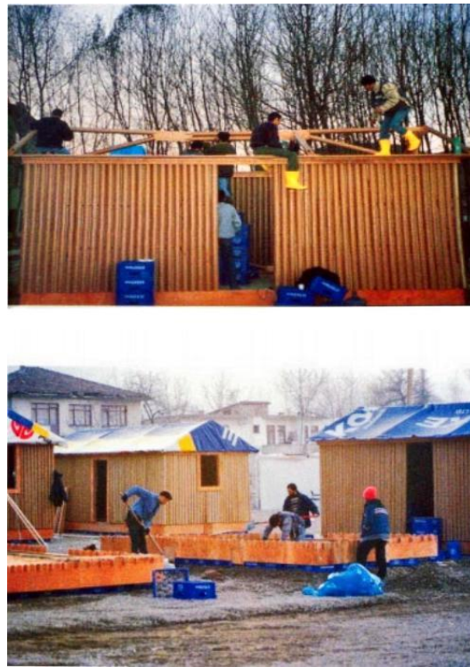
Figure 4. Relief workers preparing the floor and foundation of the paper temporary housing in Turkey.
